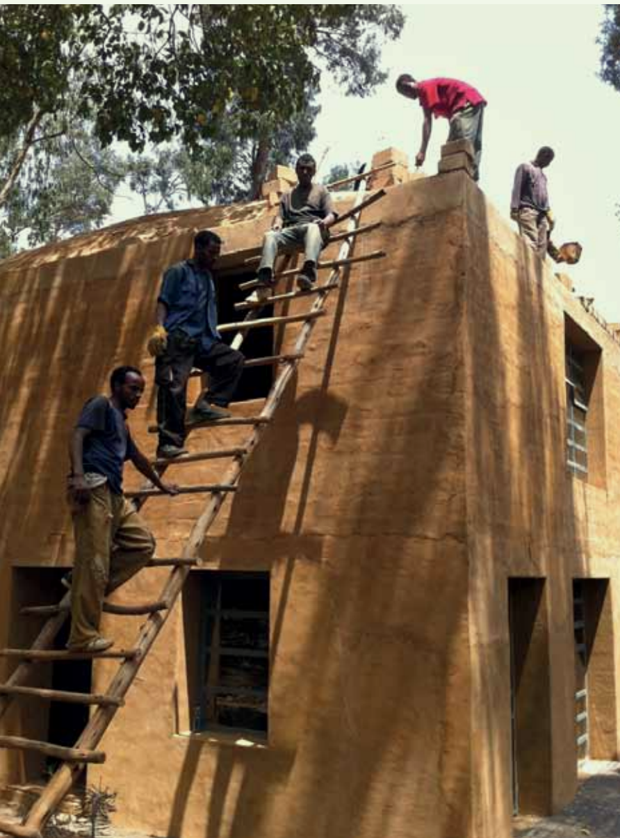
A multi-story building being constructed using local materials, Addis Ababa © BLOCK Research Group, ETH Zurich
